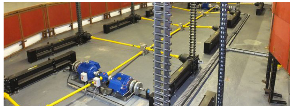
Picture 42. Derngate fixed chain lifting equipment (TV & Theatre Services)
